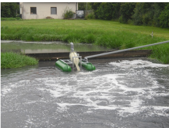
Inlet zone with simple wooden scum baffle
