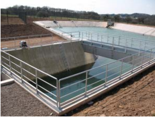
Inlet zone with scum baffle and walkway made of concrete
