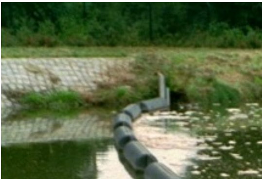
Paved inlet zone with floating scum baffle
